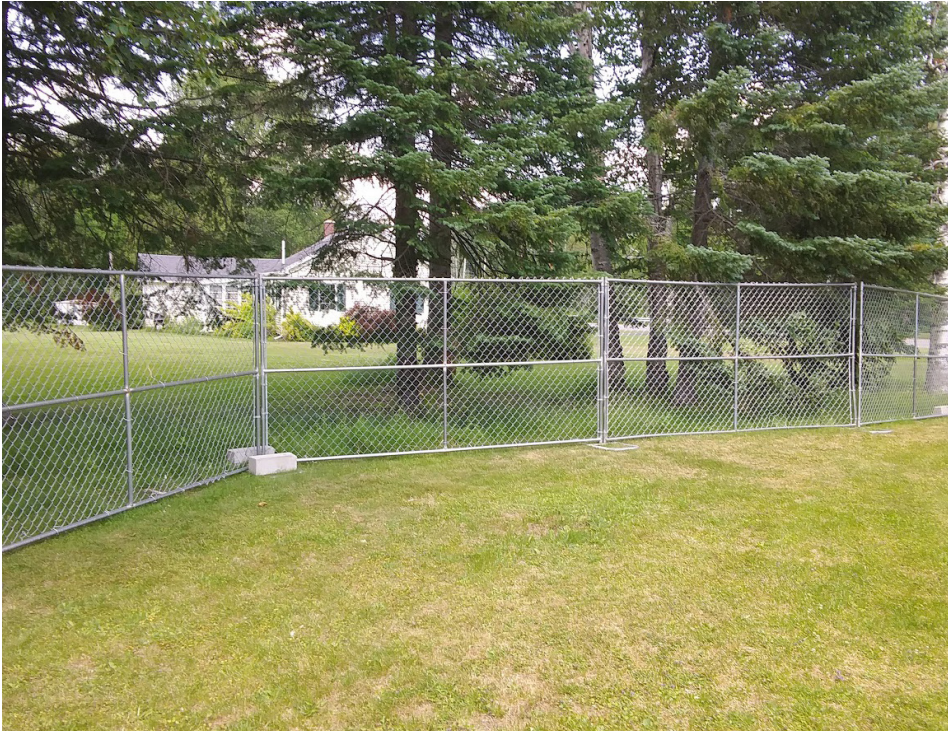
Temporary Fence with Bases
